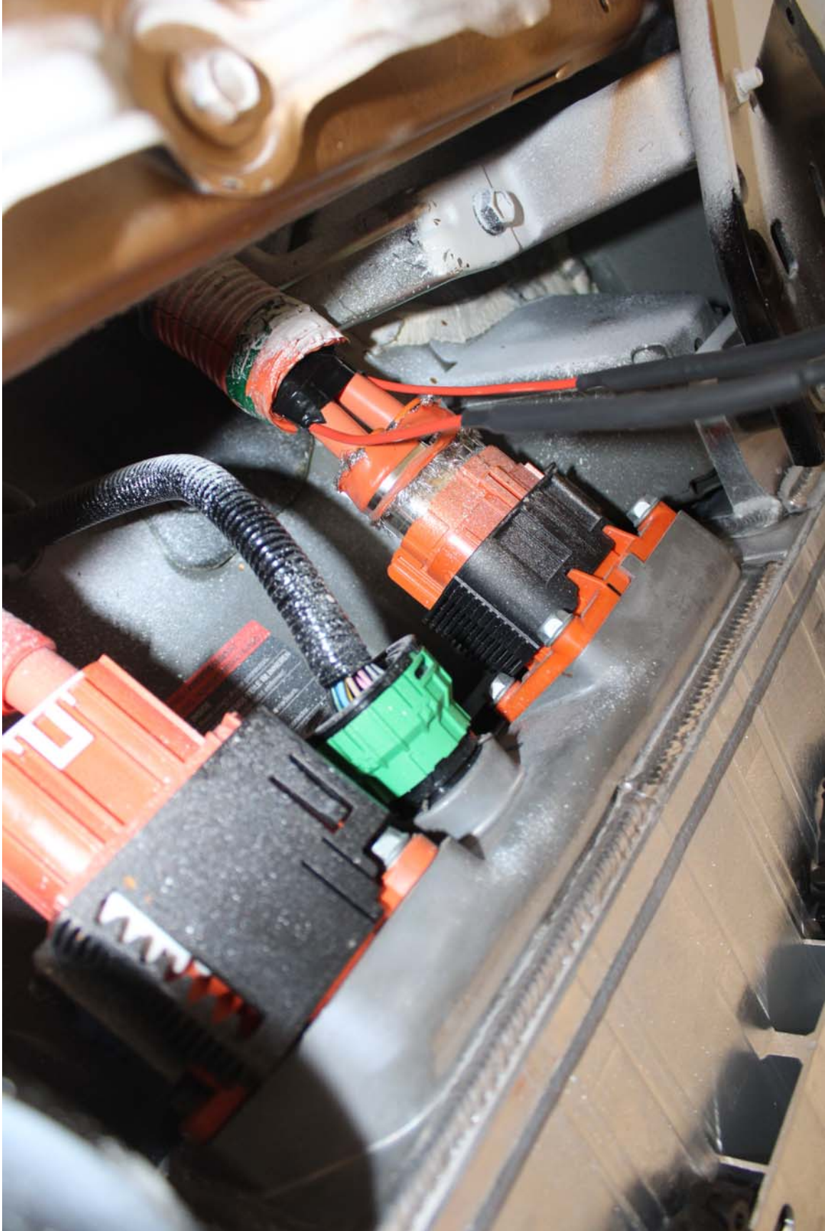
Photo No. 74. Post-Test Voltage Monitoring Leads Attached to Electric Energy Storage System
