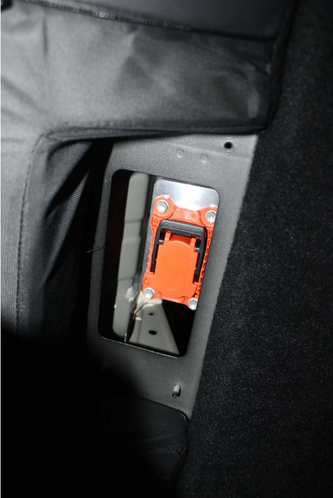
Photo No. 69. Pre-Test Manual Service Disconnect in Place
