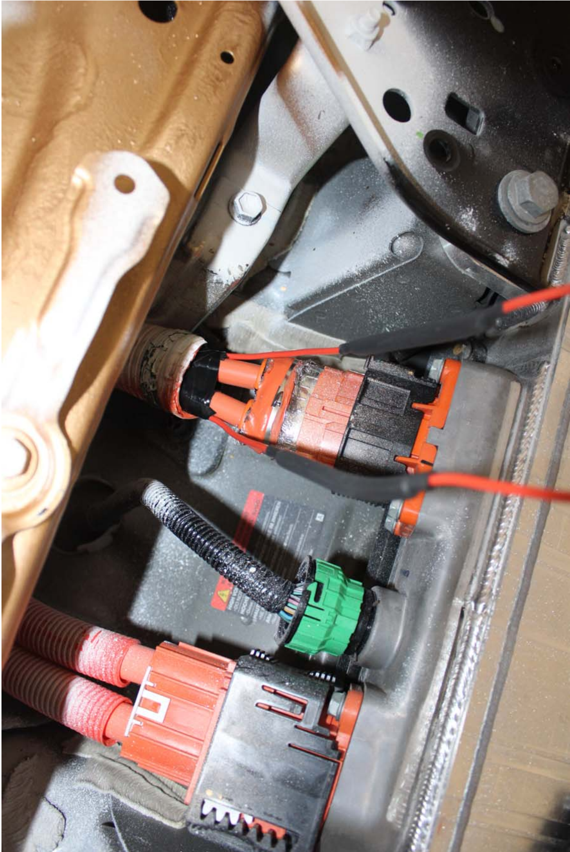
Photo No. 73. Pre-Test Voltage Monitoring Leads Attached to Electric Energy Storage System
